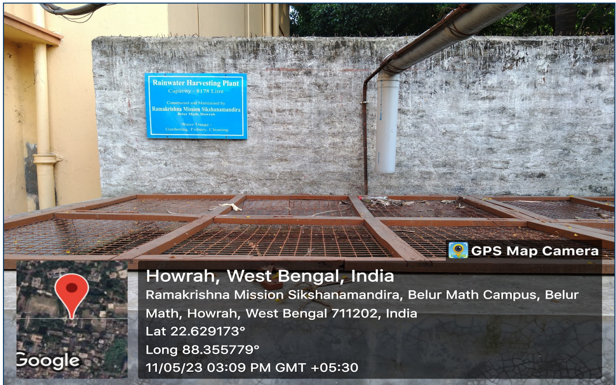
Rooftop Rain water harvesting at Ramakrishna Mission Sikshanamandira
