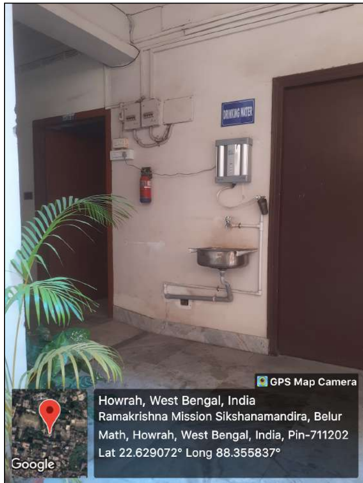
7.3 Drinking Water Facilities with Purifiers at Ground Floor.
