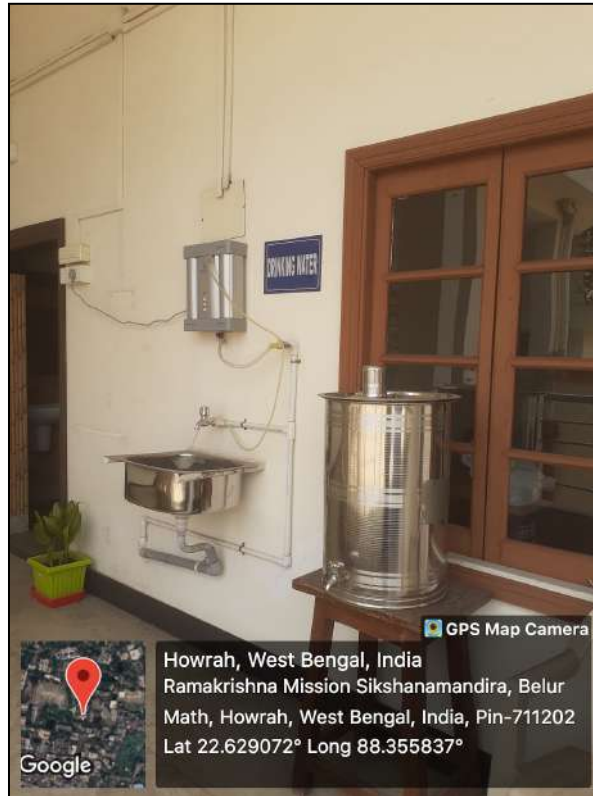
7.1 Drinking Water Facilities with Purifiers beside the Nivedita Hall (Third Floor).
